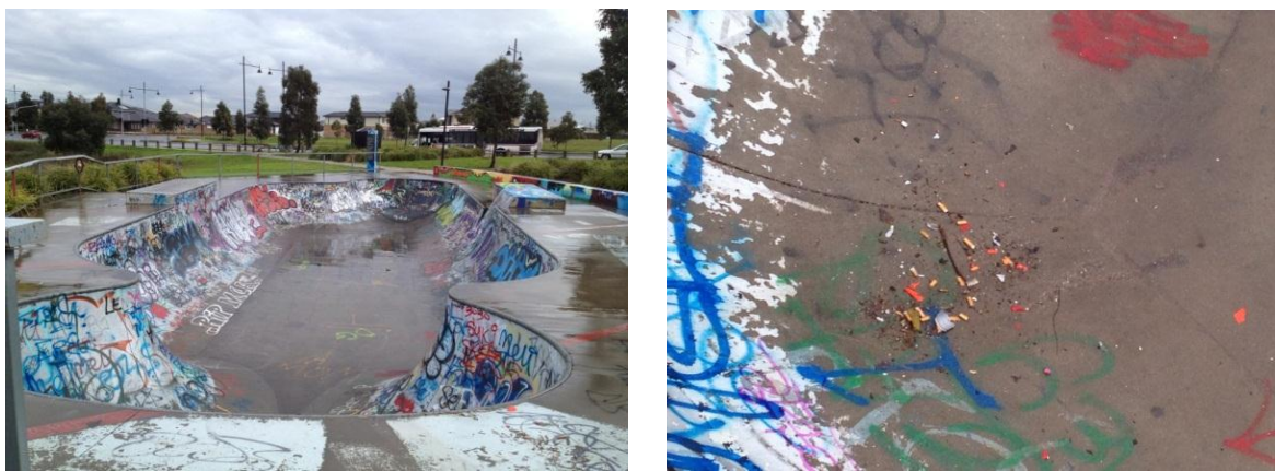
Figure 10: Overall view of the bowl showing significant graffiti & some litter collecting in the bowl with minor pock marks.
