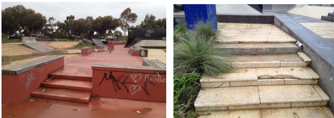
Figure 14: Photo shows some graffiti present around the park and a view of broken pavers in stepped viewing area that need replacement.
