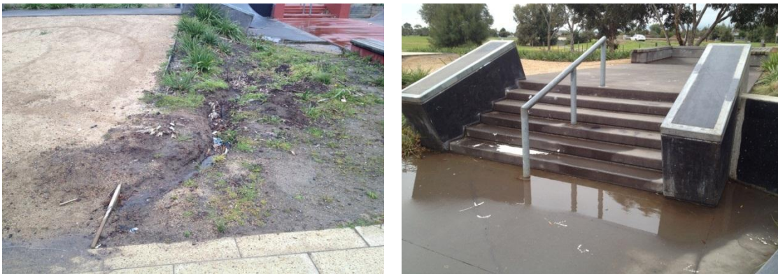
Figure 15: Photos showing embankment eroding with water and flooding and evidence of flooding at the base of a set of stairs that creates a significant hazard
