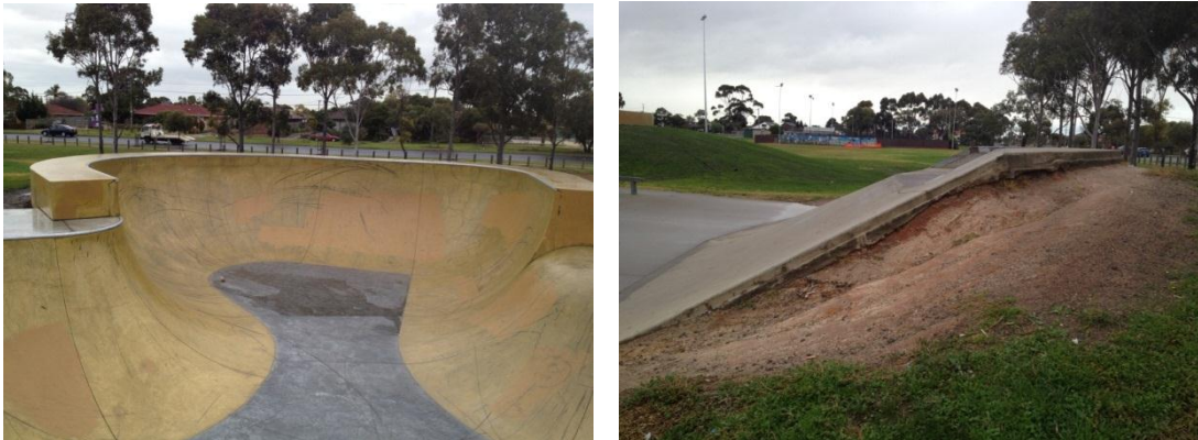
Figure 12: View of brand new bowled section neat and well integrated into the rest of the park. Along most edges though of the older areas, there is significant wear to the batters exposing the slabs as the second photo shows.
