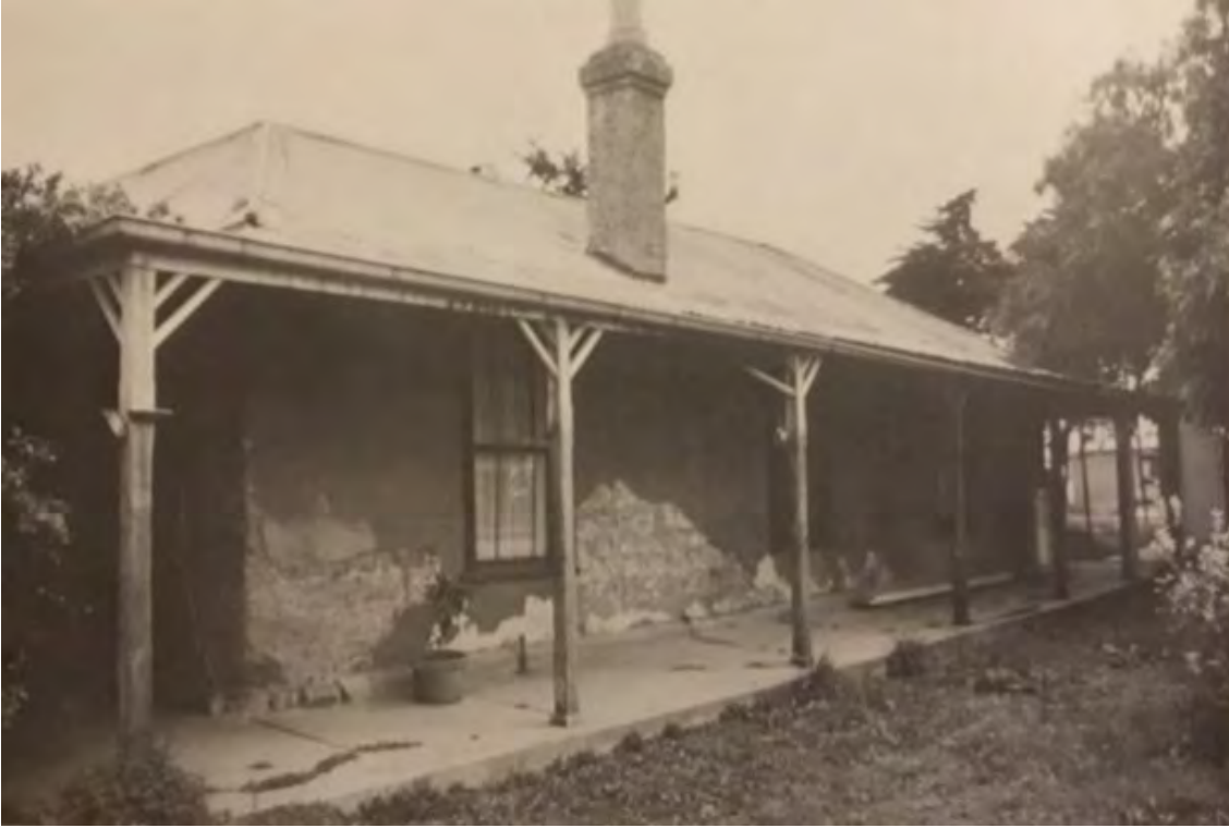
Figure 19 Early farmhouse of William Ison on Bulban Road, Werribee, was constructed of adobe. Source: Miles Lewis, Victorian Primitive , 1977, p. 36; photograph by Miles Lewis
