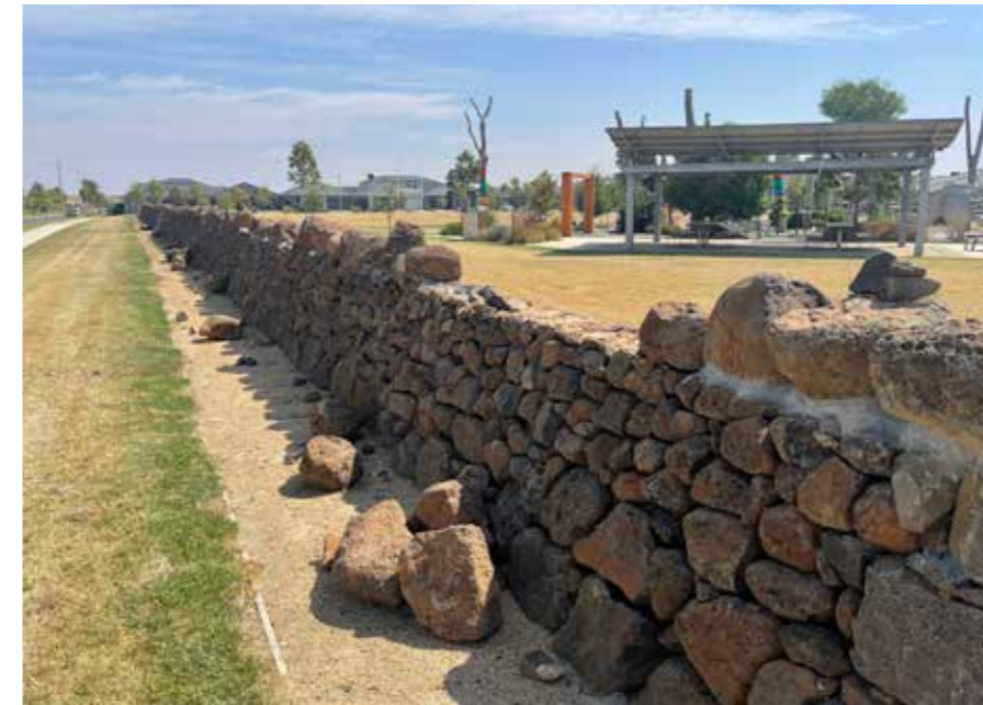
Figure 29 Photograph of the dry stone wall, facing west. Note the dislodged cope stones and inappropriate use of mortar. Source: Wyndham City Council
