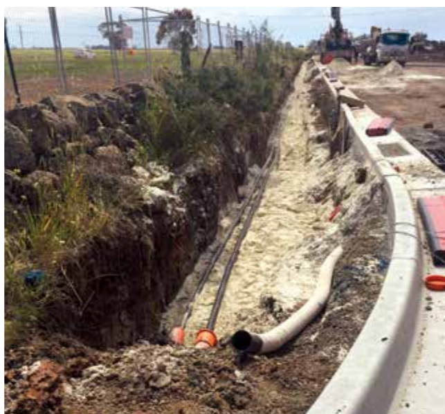
Figure 23 Infrastructure works occurring too close to dry stone walls create an unsafe working environment.
